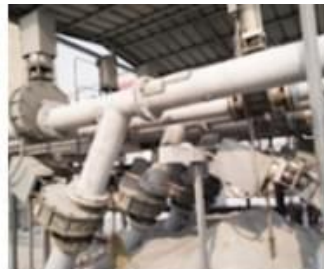
prone to cracks
